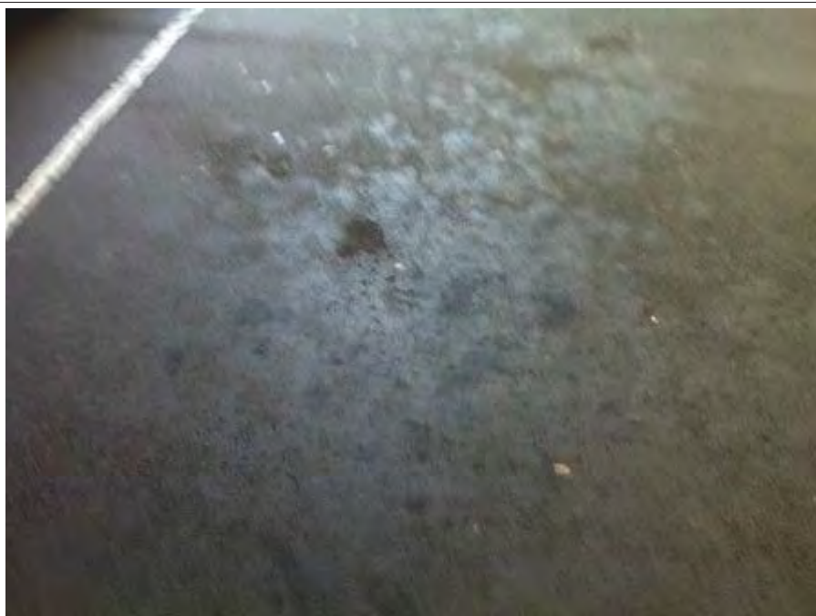
Photo 5.8.1 – Example of oil spotting on the surface of the asphalt in the undercroft parking area
