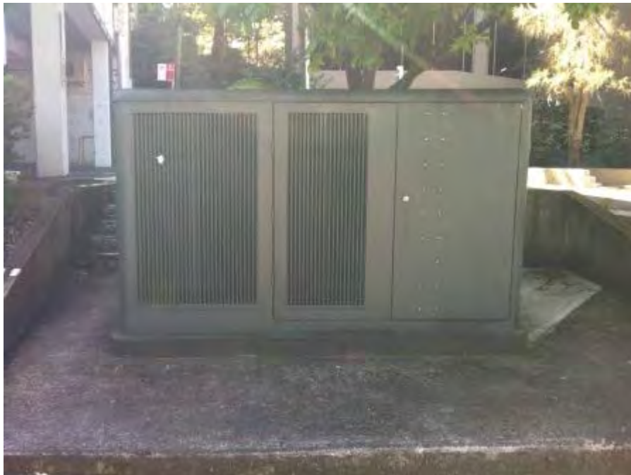
Photo 5.1.1.7 – Electrical kiosk located adjacent to south western corner of council administration building
